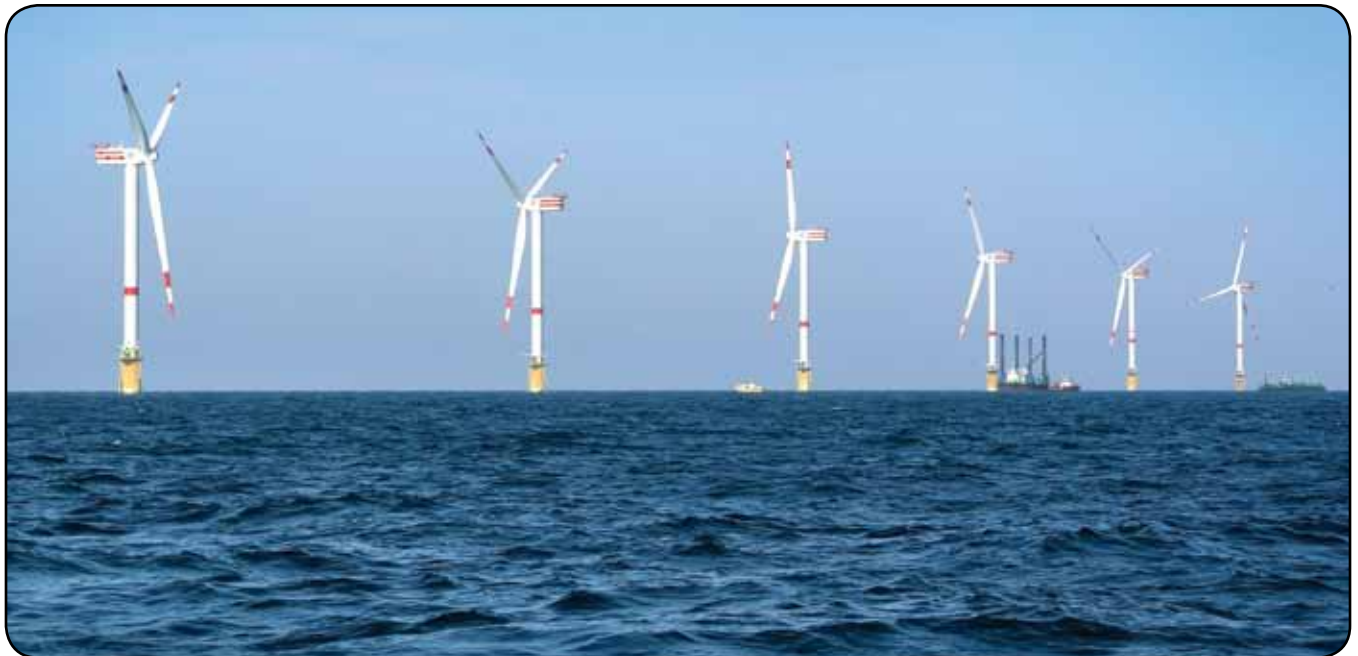
This photo captures the final phase in the construction of wind turbines on the Thornton Bank in September of 2008. The turbines are situated 17 miles off shore, on the Belgian portion of the North Sea. Photo © Hans Hillewaert.
